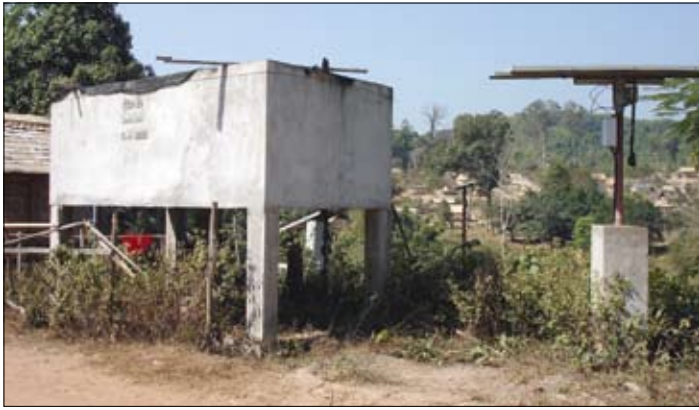
Water tank with PV-operated pump in Ban Sorge (Laos)
