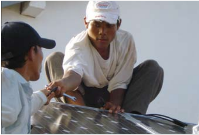
Installation of PV systems for the orphan houses in Khamphong Thom (Cambodia)
