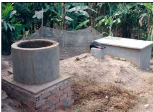
Small biogas plant in operation (Cambodia)
