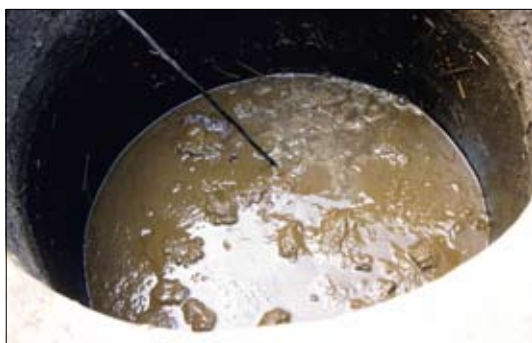
Mixing pit for anaerobic digestion processes
